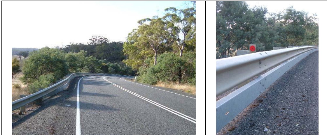
w-beam safety barrier with 'rub rail', Tasman Highway, west of Buckland
