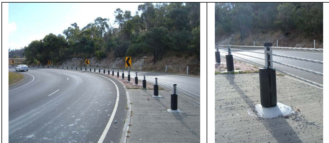
Wire rope safety fencing with 'stack cushions', Tasman Highway, eastbound off-ramp to Mornington interchange
