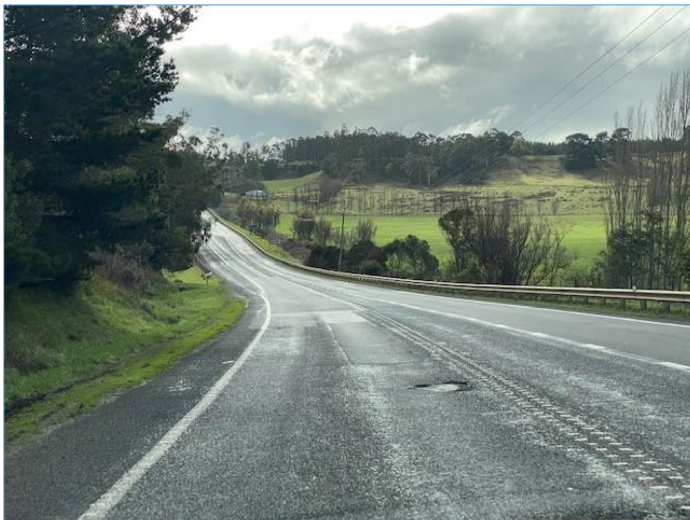
Figure 6.3: Pothole near the Parramatta Creek Rest Area
