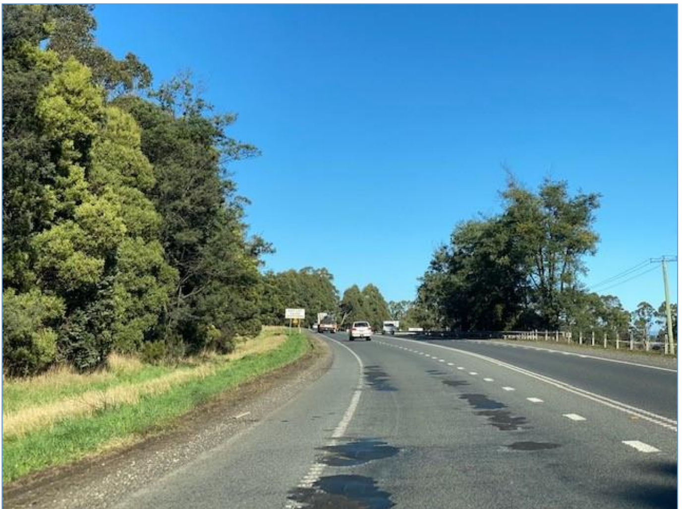
Figure 4.8: Pavement near Elizabeth Town showing localised pavement patching
