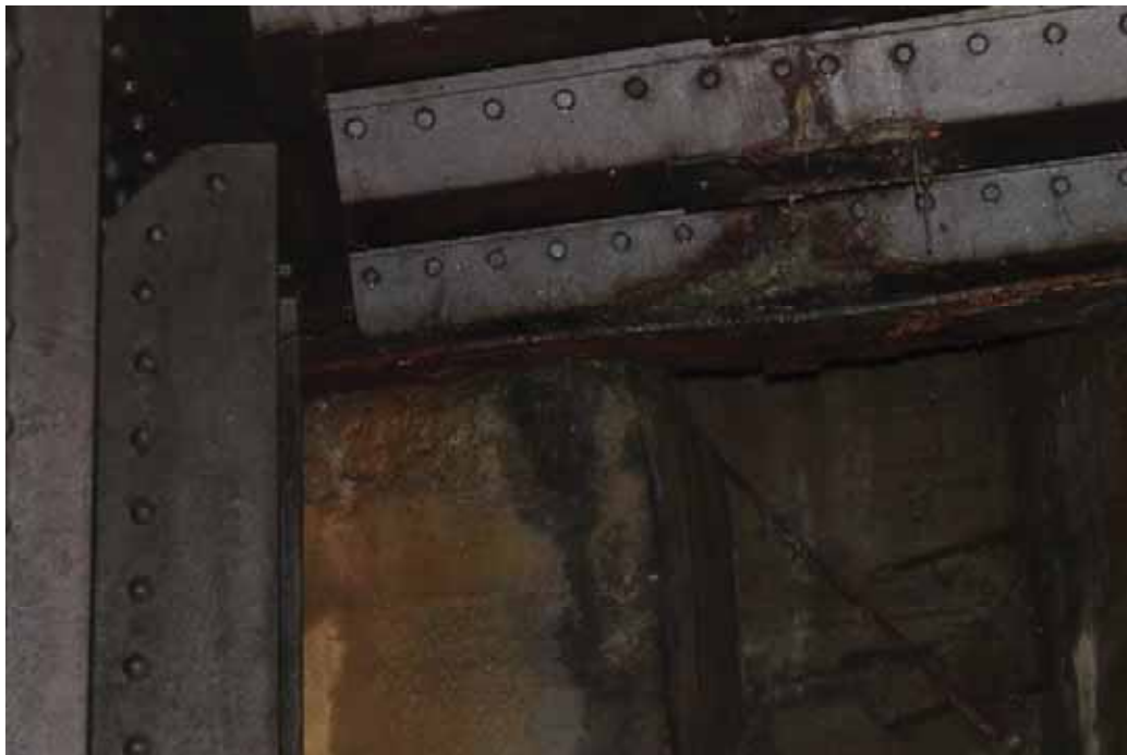
Figure 10 Deflection in Deck 2 end member with corrosion (typical)
