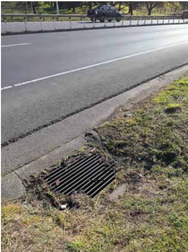
Photo Inlet – pit adjacent to the footpath appears to flow towards pit along the road
