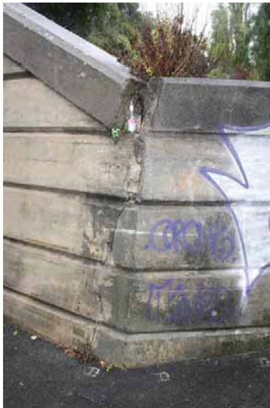
Figure 12 Major cracking at interface between wingwall and wingwall return with spalling
