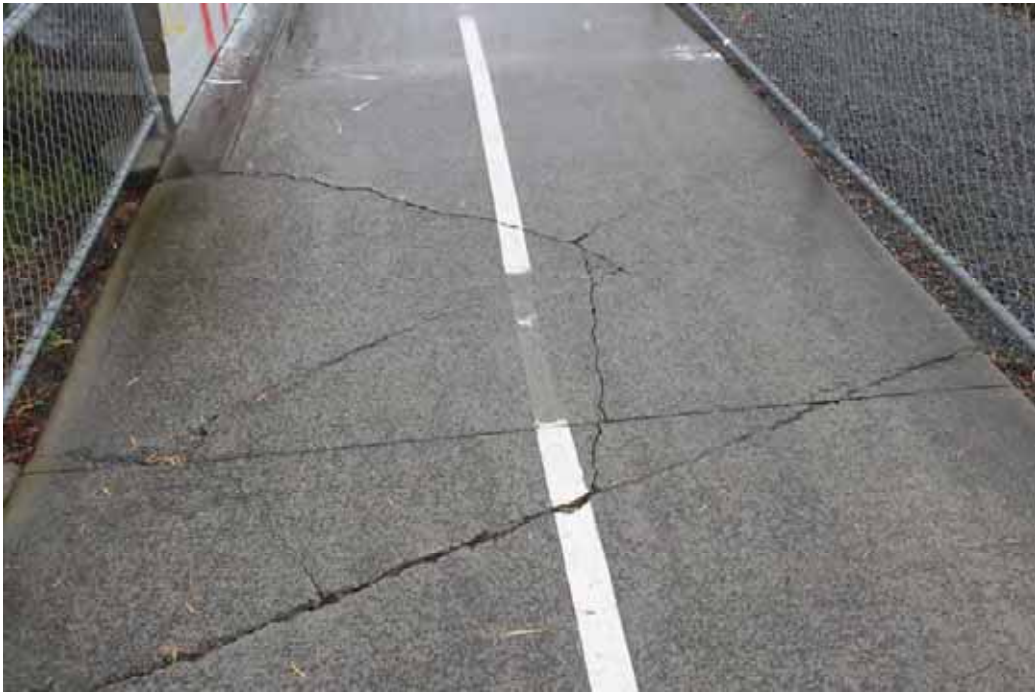
Figure 5 Failure of footpath concrete at Approach 1 (typical)
