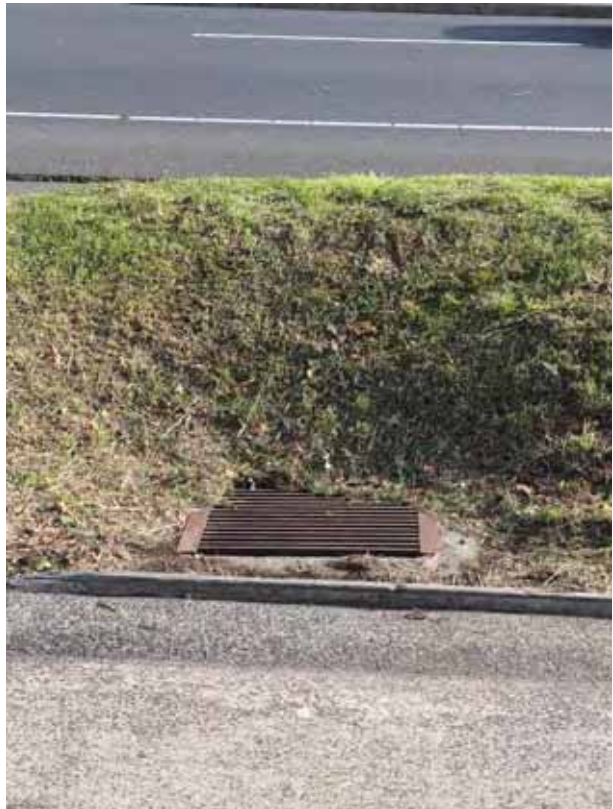
Photo Inlet – adjacent to the footpath
