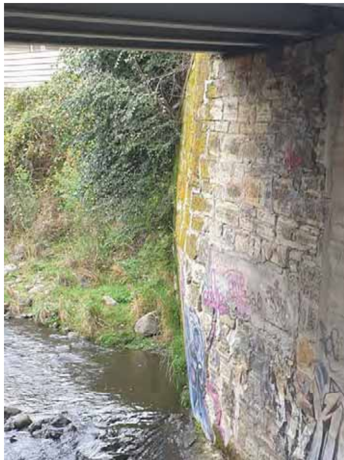
Figure 6 Bulging in the sandstone wall at Abutment 2
