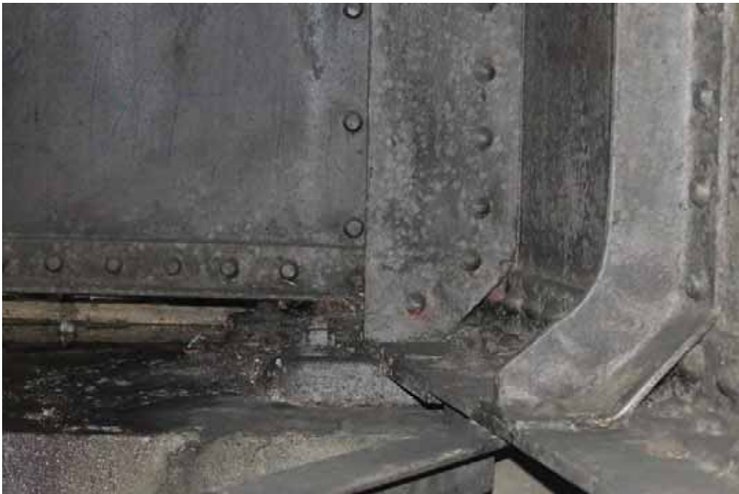
Figure 8 Build-up and moisture at bearing (typical)
