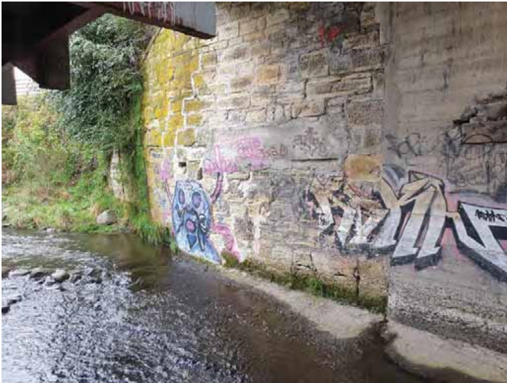
Figure 5 Deteriorated sandstone wall and wingwall movement at Abutment 2
