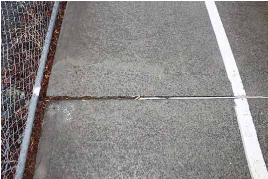
Figure 6 Joint Failure at Abutment 2
