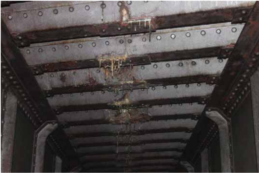
Figure 11 Stalactites on deck soffit (typical)
