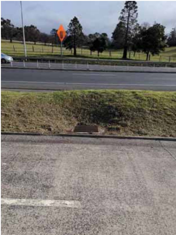
Photo Inlet – adjacent to the footpath
