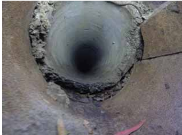
Photo Inlet – upstream side
