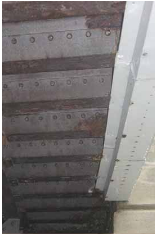
Figure 9 Corrosion extending from steel flashing at Deck 3 (typical)
