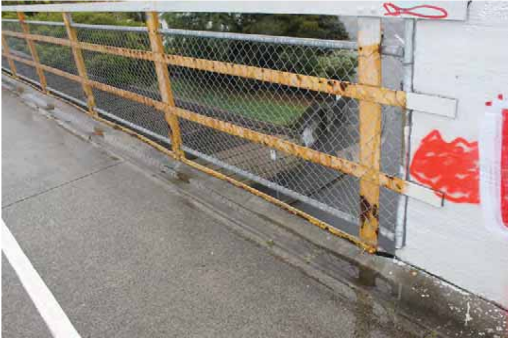
Figure 7 Guardrail 1 with corrosion and deflected kick plate (typical)
