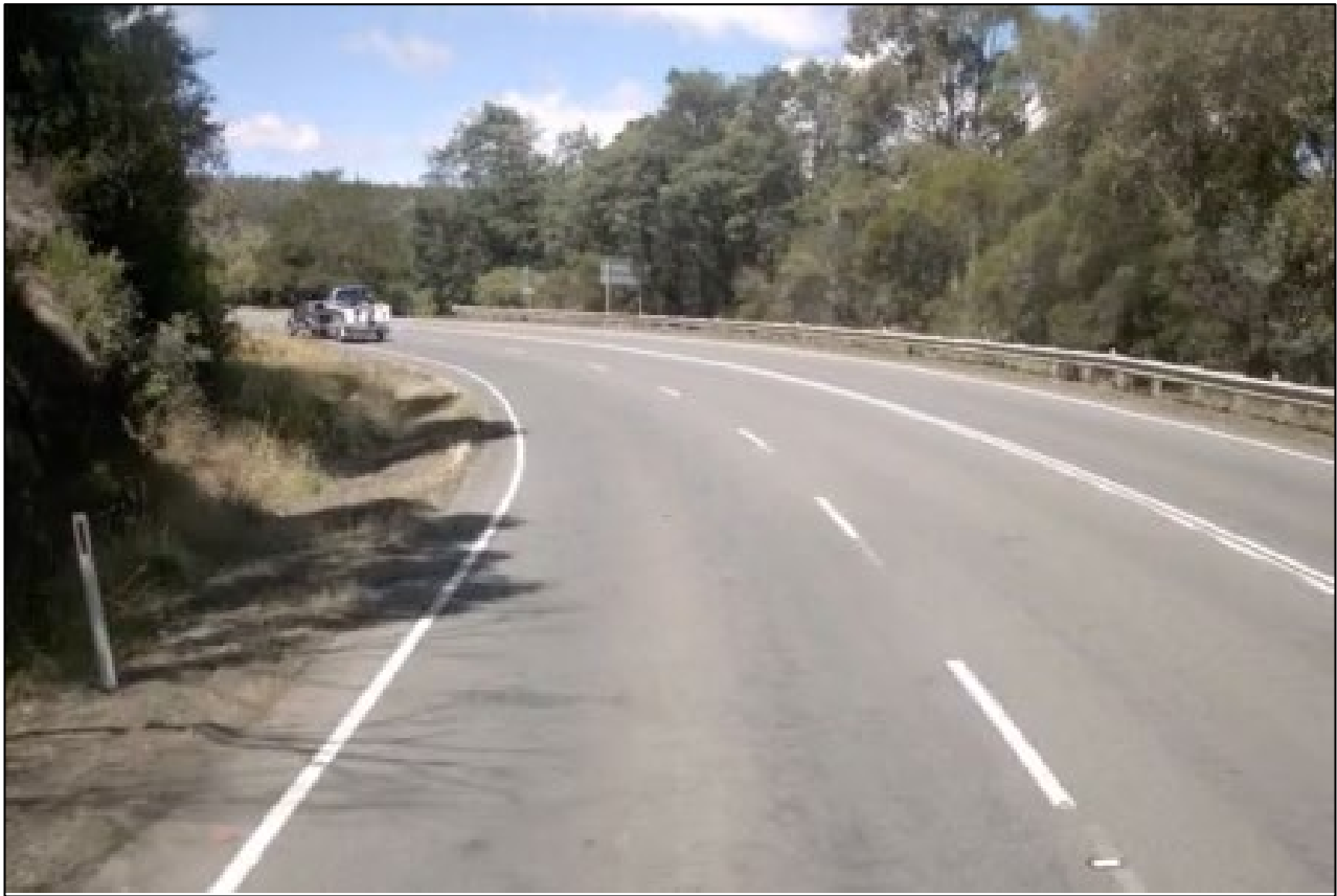
Figure 4-13: Pavement deformations near Kyalami corner, Lower Longley
